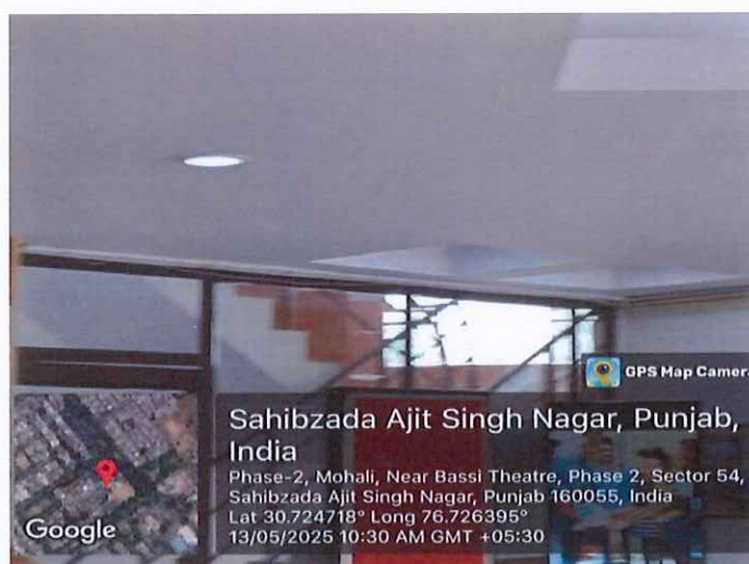
LED Bulbs installed across campus
