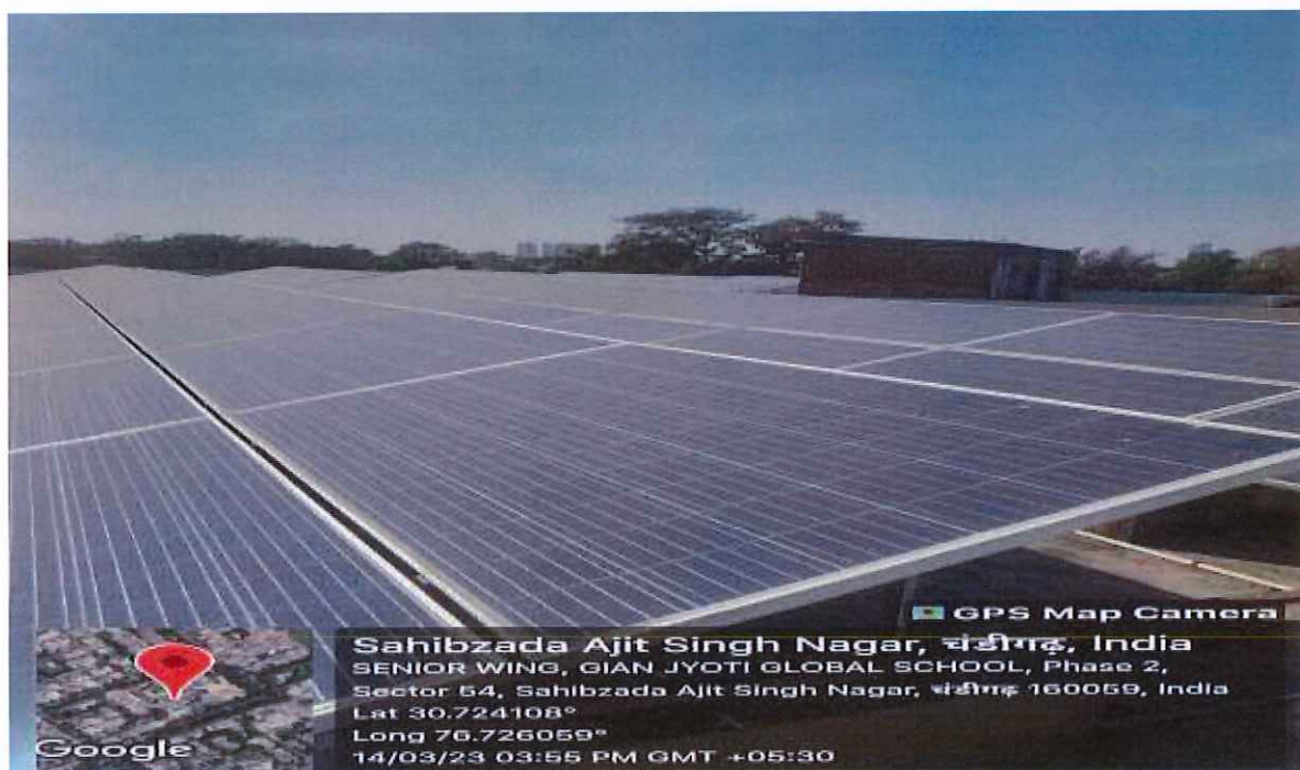
Solar Power plant (200 KWP) installed in campus
