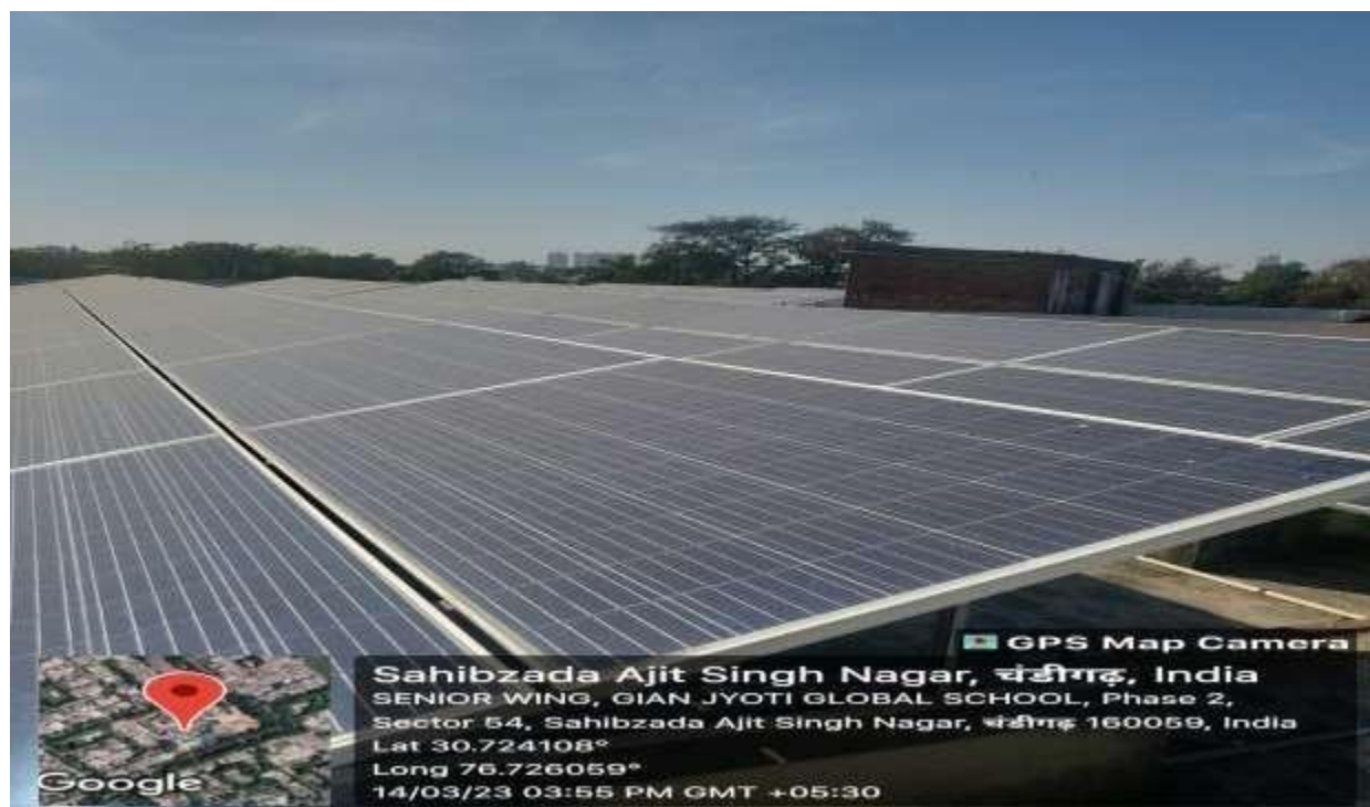
Solar Power plant (200 KWP) installed in campus
