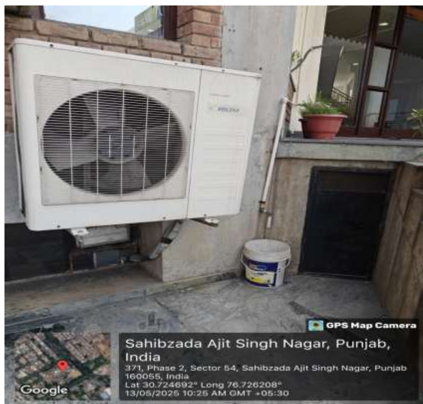
AC condensate water collected in buckets for gardening and sanitation use on campus
