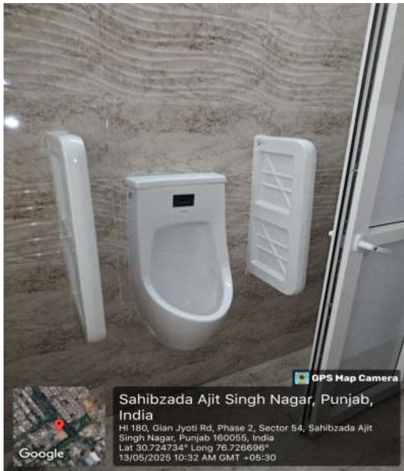
Urinal Sensor Flusher installed in Washroom
