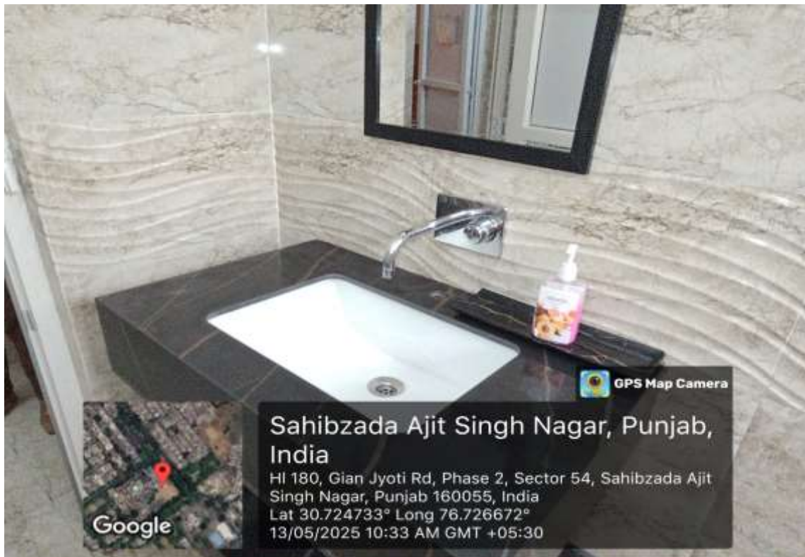
Pressmatic taps installed in Washroom
