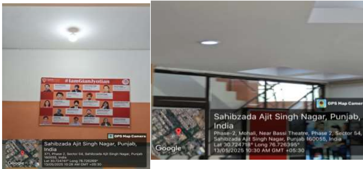
LED Bulbs installed across campus
