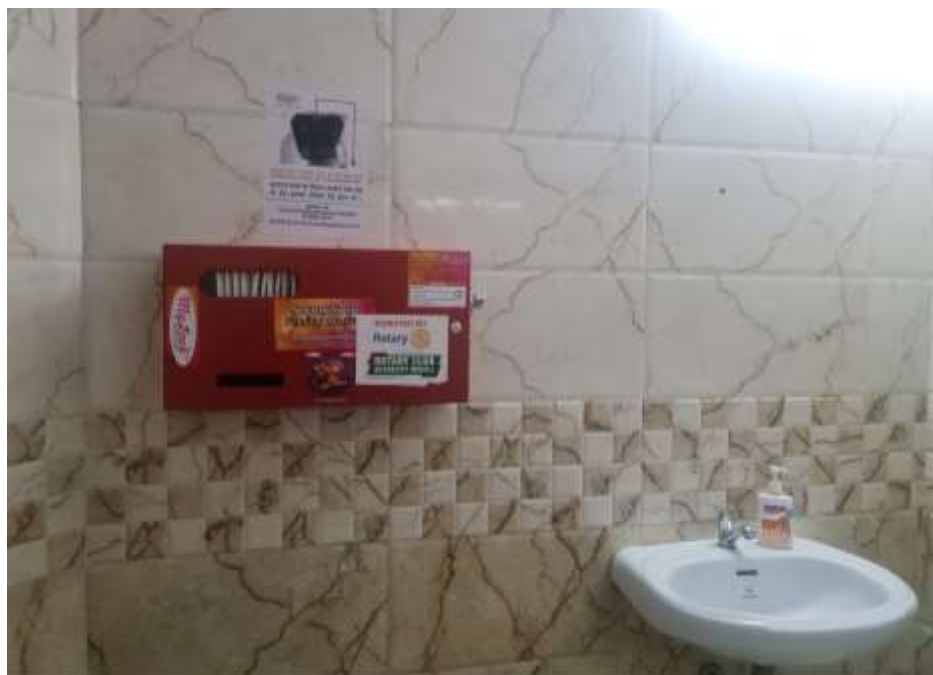
D. Installation of Sanitary Pad Vending Machines
