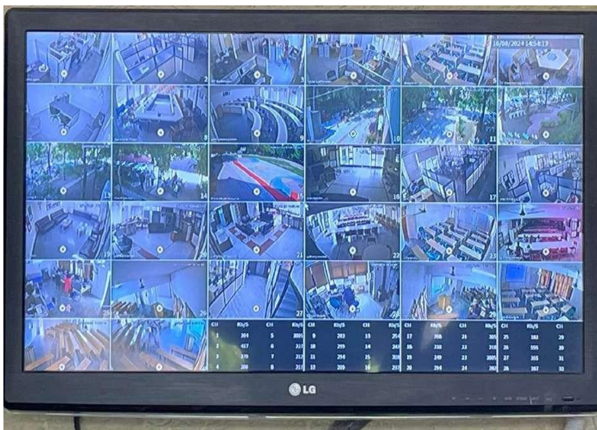
CCTV Surveillance View from the Director's Cabin, GJIMT
